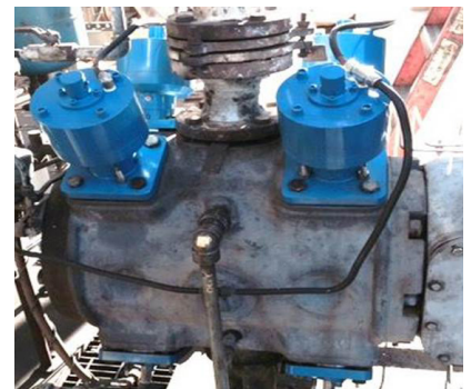
CPI plug unloader actuators with upgraded seals which reduced their emissions and improved reliability
