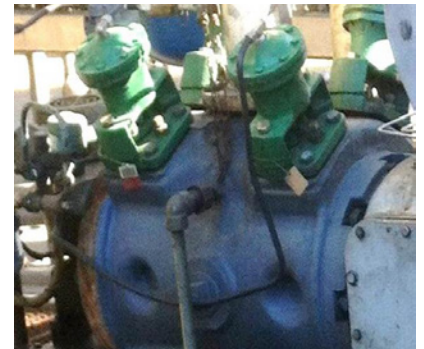
A refinery customer experienced problems with gas leakage from their OEM old style diaphragm unloader actuators
